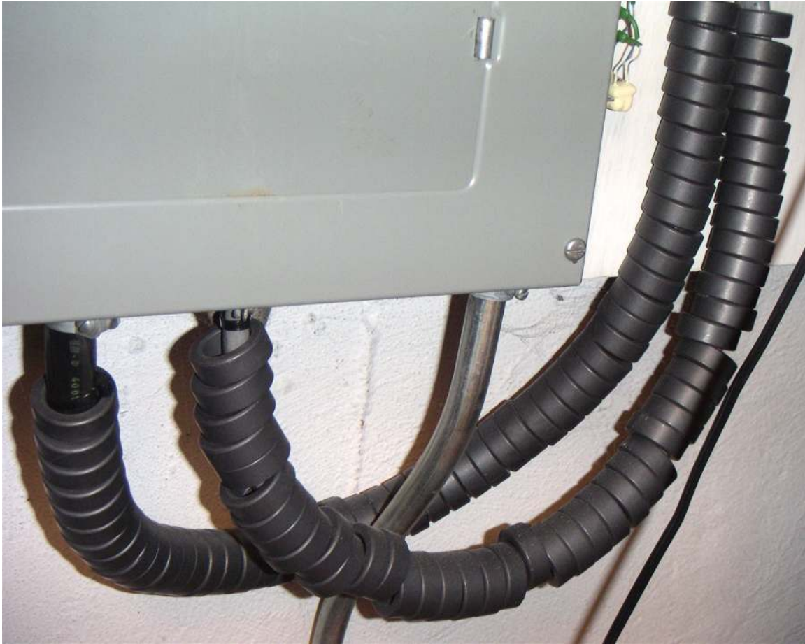
Figure 14: Common-mode chokes formed by stringing ferrite toroids like beads on two 3-conductor, 240-VAC power cables, one 60-A and one 40-A.
